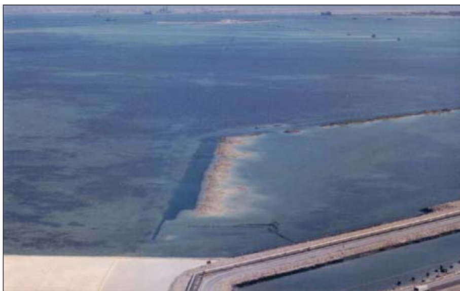
This photograph shows the path of the trenching works from WVS to QAQ Island (Fig. 5).
