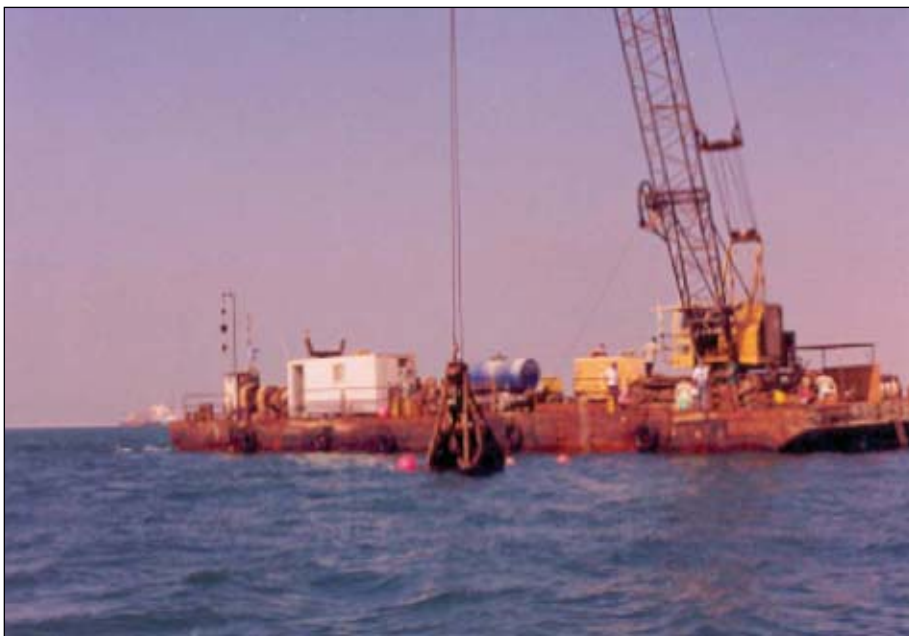
Bapco excavated trenches between WVS and QAQ Island using this marine channel trenching barge (Fig. 6).
