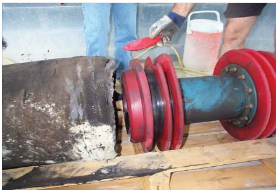
Excavation retrieved a soft-form pig and conventional bidirectional pig caught inside the damaged pipeline (Fig. 9).
