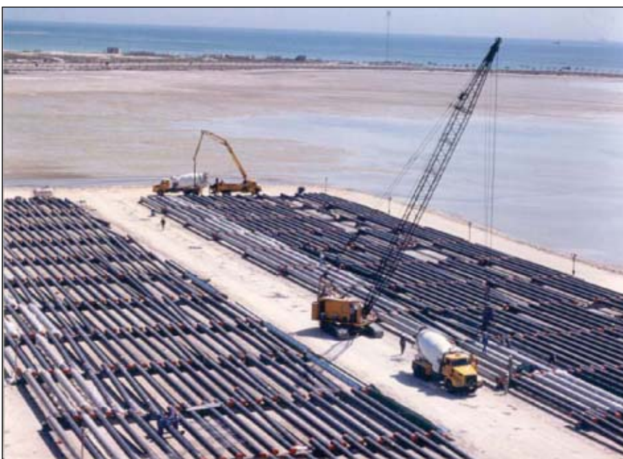
Bapco welded pipe joints into 348-m lengths at this onshore fabrication yard. A total of 51 strings was fabricated and installed (Fig. 3).
