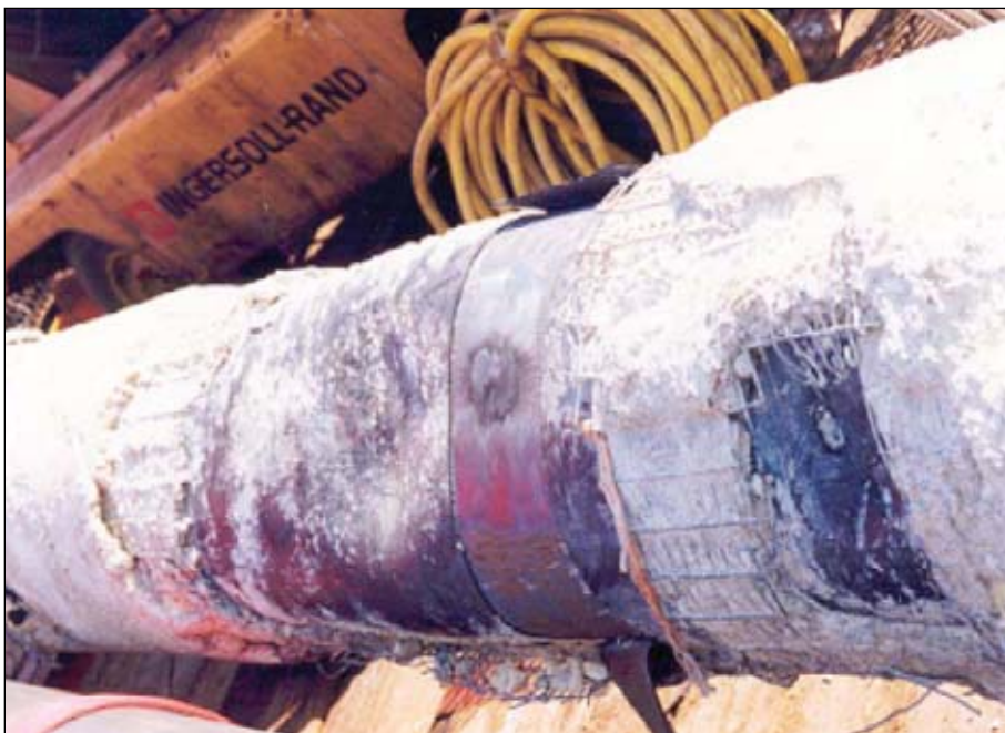
Bapco cut the damaged length of pipe (shown here) out of the pipeline and replaced it with good pipe (Fig. 10).
