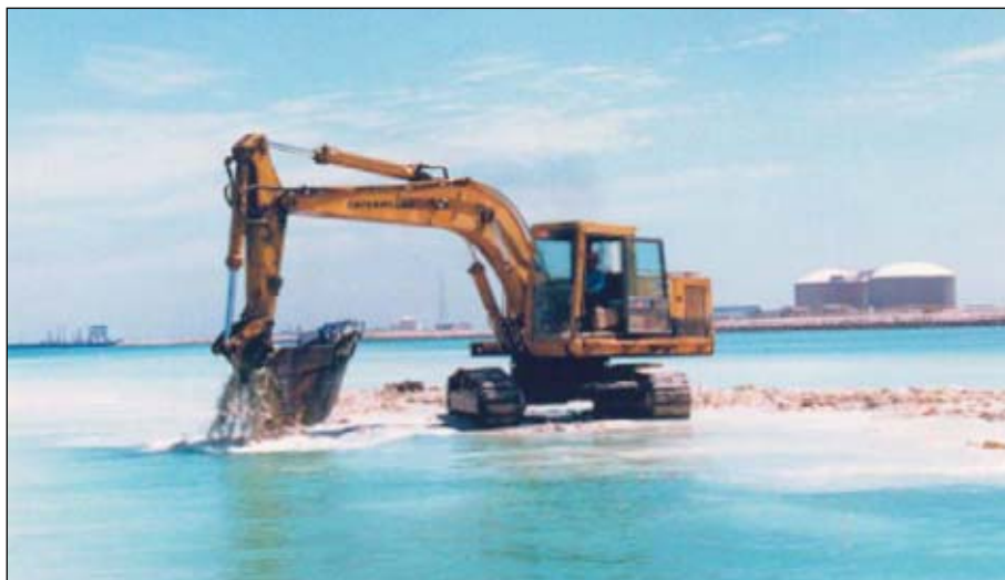
Excavation of the trench from the wharf valve station across QAQ Island used tracked excavators, working during daylight at low tide in the offshore areas. The excavators created their own causeways using excavated fill (Fig. 4).
