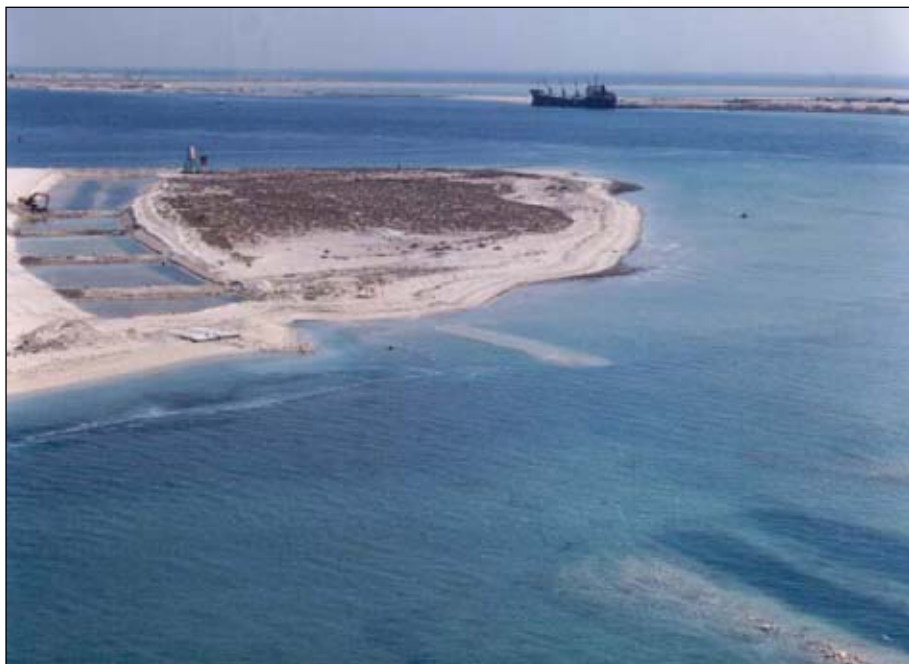
Trench crossing the 10-in. gas pipeline at the southern portion of QAQ Island required care in its execution (Fig. 7).
